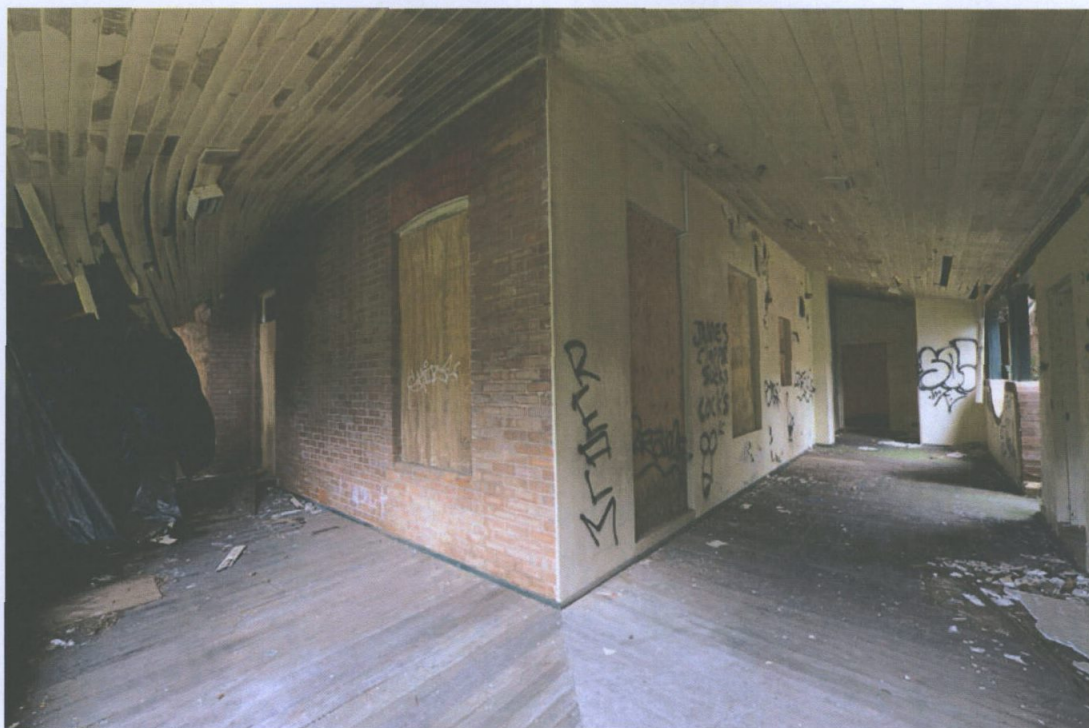
Figure 12 View along west/south verandahs showing verandah roof collapse, vandalism and the remains of rendered walls from the rear verandah enclosure. Paul Davies 2014.
