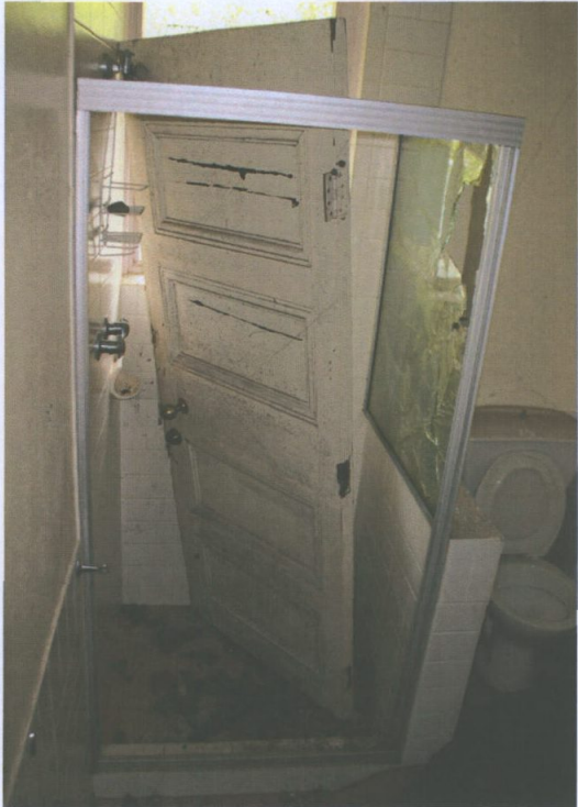
Figure 23 Bathroom in former garage with vandalised original door. Paul Davies 2014.
