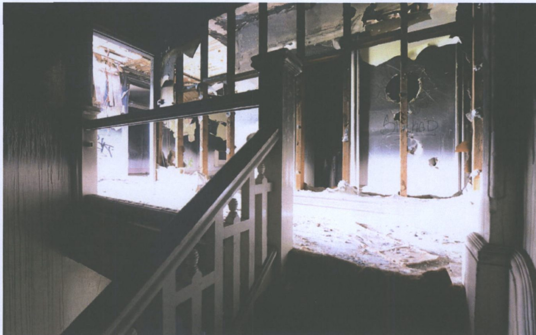
Figure 25 Stairway to second floor facing northwest. Note later timber framed walls that have been burnt and vandalised. Most of the immediate fire damage is superficial with the stair and its enclosure remaining structurally sound. The stair has undergone substantial vandalism. Paul Davies 2014.
