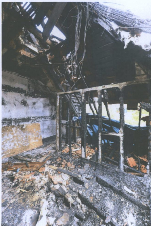
Figure 26 Room 17, including overview of fire damage. Paul Davies 2014.
