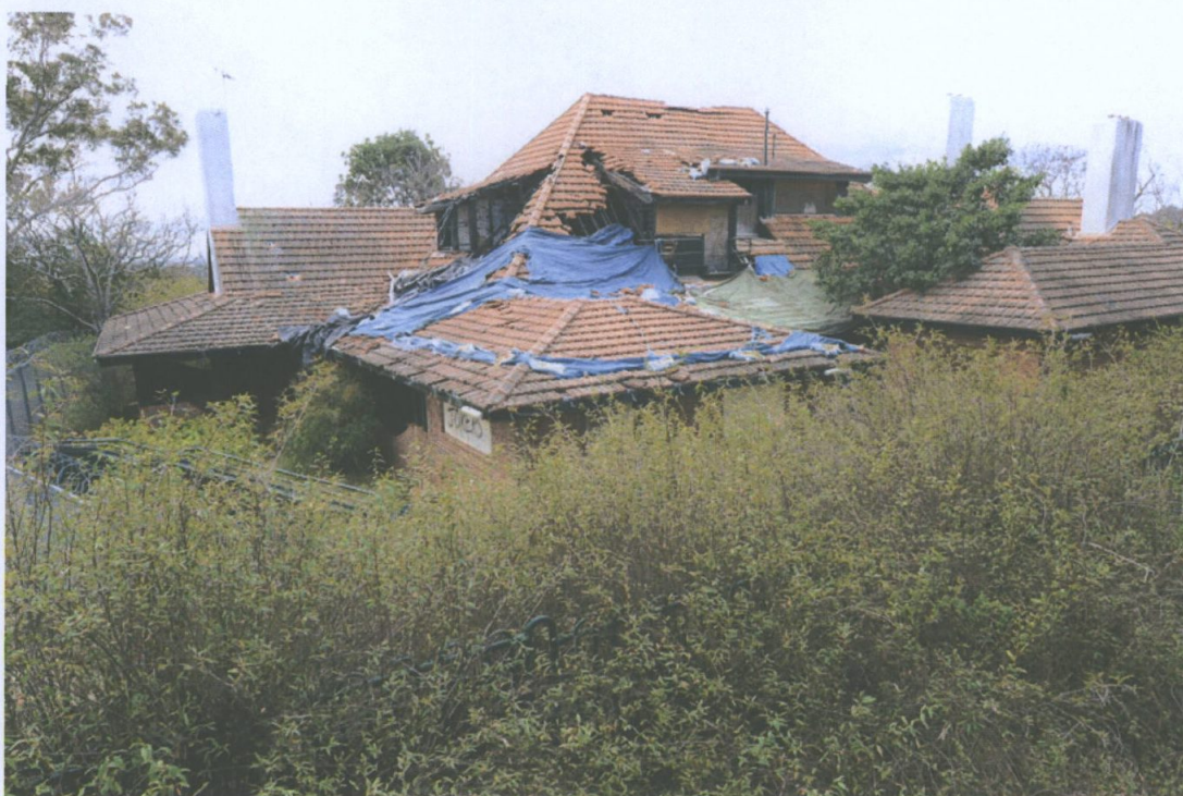
Figure 31 Overview of house from west of rear embankment. Apart from fire damage the photo shows the poor quality of planting on the bank and the need to consider a landscape treatment for the area that provides separation between adjacent uses and enhances the setting of the house. The child-care facility will retain overviews as it is elevated even with significant landscape treatment. The boundary fence can also be discerned in the foreground as a green metal fence. Paul Davies 2014.
