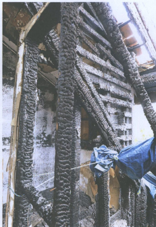
Figure 27 Room 17, including detail of fire damage. Paul Davies 2014.
