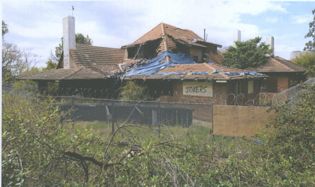
Figure 34 View from the west. This further demonstrates the potential to add some discrete additions to the rear of the building. Paul Davies 2014.
