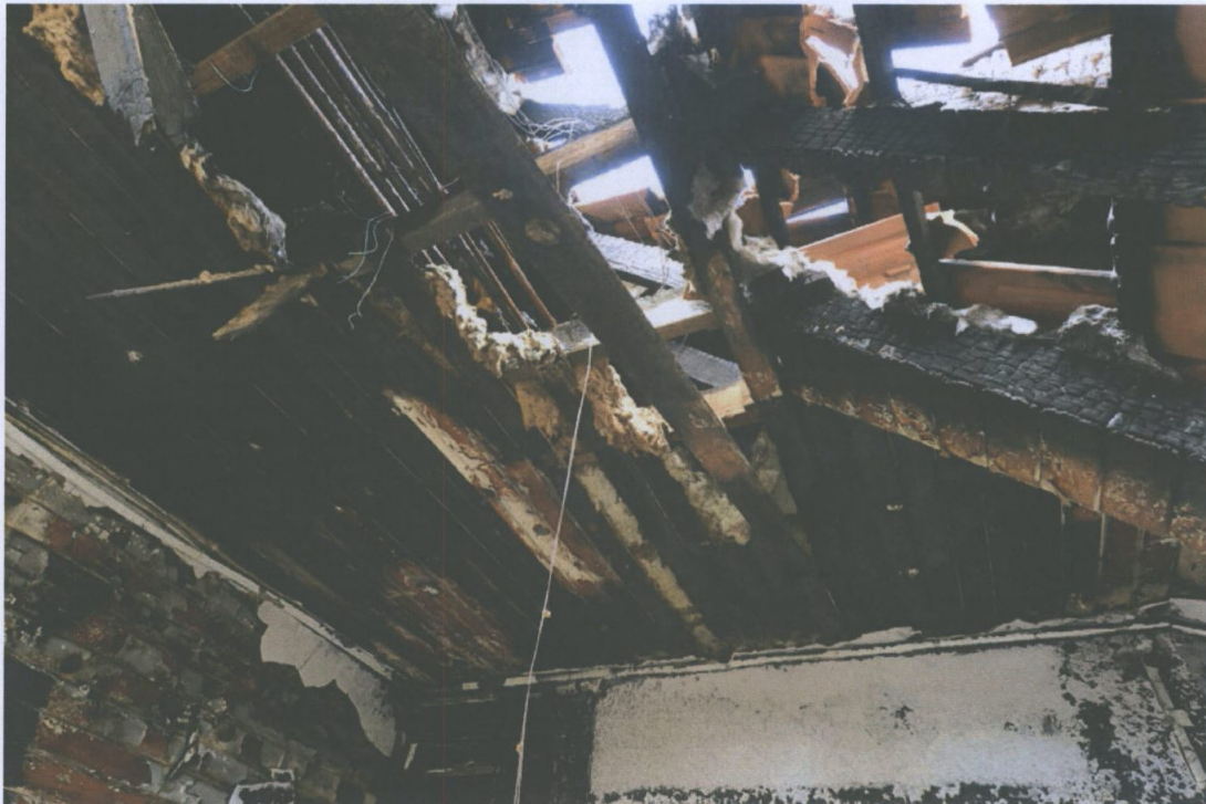
Figure 28 Room 17 roof area showing fire damage. Paul Davies 2014.
