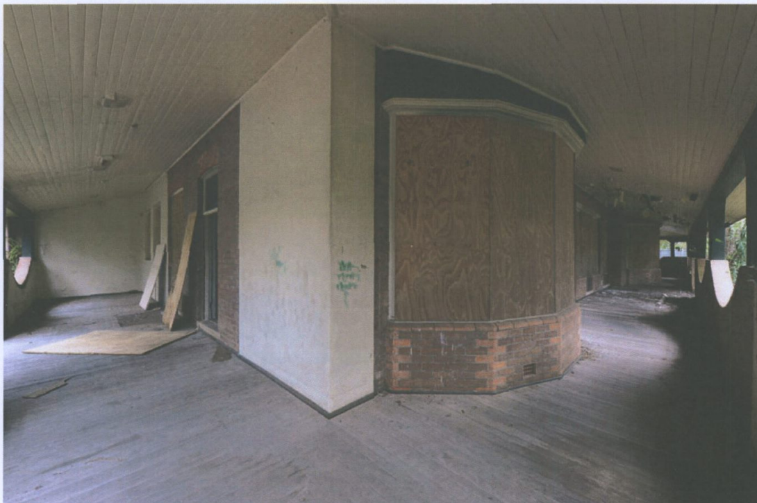
Figure 10 View along the verandah of both the eastern and northern façade. Note the rendered walls where earlier verandah enclosures were created. Paul Davies 2014.
