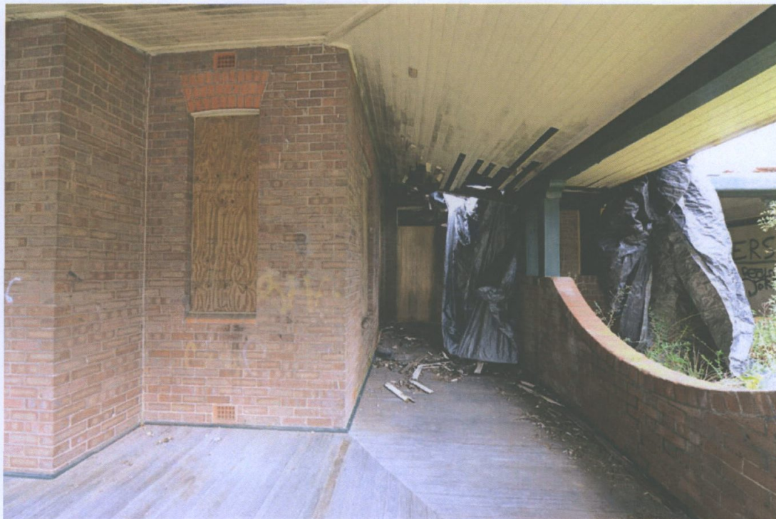
Figure 11 View along the western verandah showing roof damage. Paul Davies 2014.
