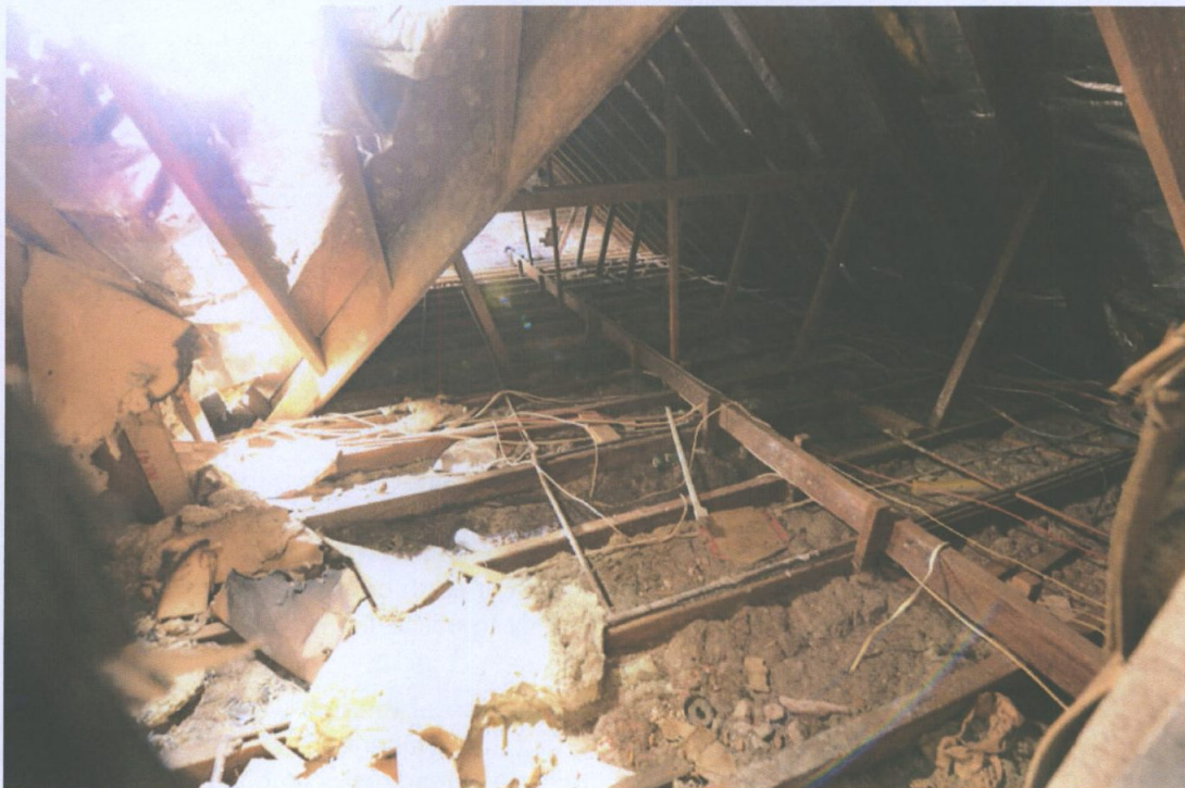
Figure 29 Interior of roof void over main reception room, generally the roof in this area has remained without damage, however it requires cleaning and tile repair above. Paul Davies 2014.
