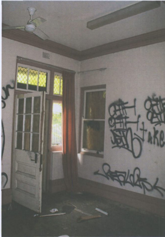
Figure 17 Room 11 facing southeast. This room was originally two small staff bedrooms accessed only from the exterior doors. The window to the right is a later addition. Paul Davies 2014.
