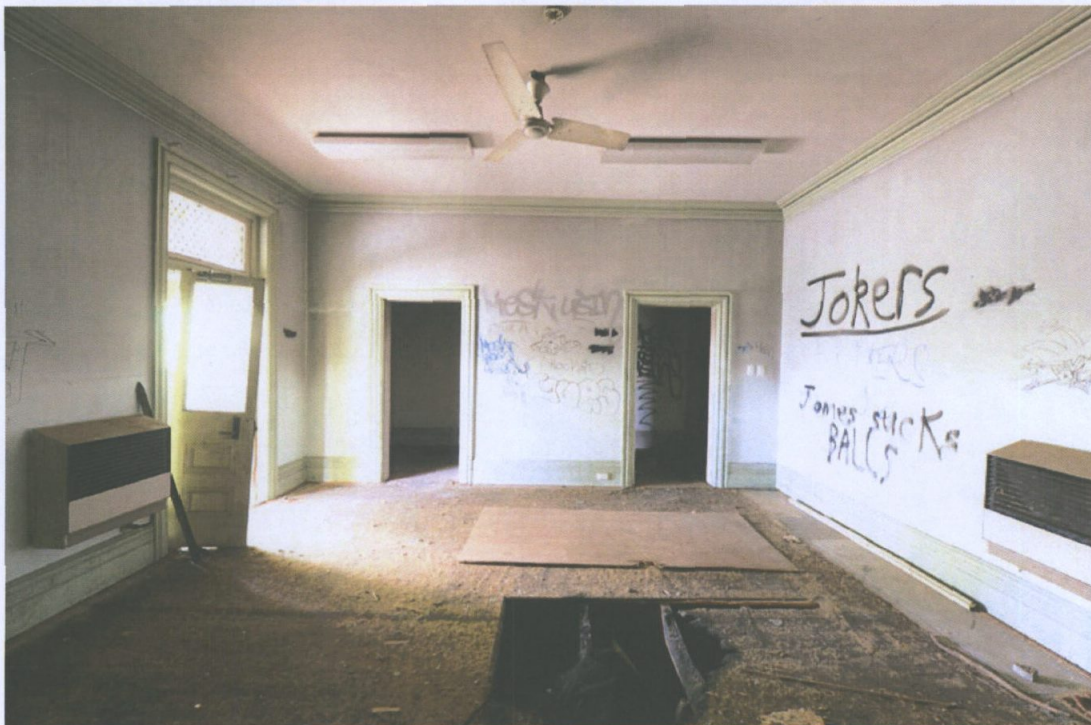
Figure 14 Main Living Room with vandalism damage, fire damage and the later fitout of plaster ceiling, heaters and fans. Paul Davies 2014.
