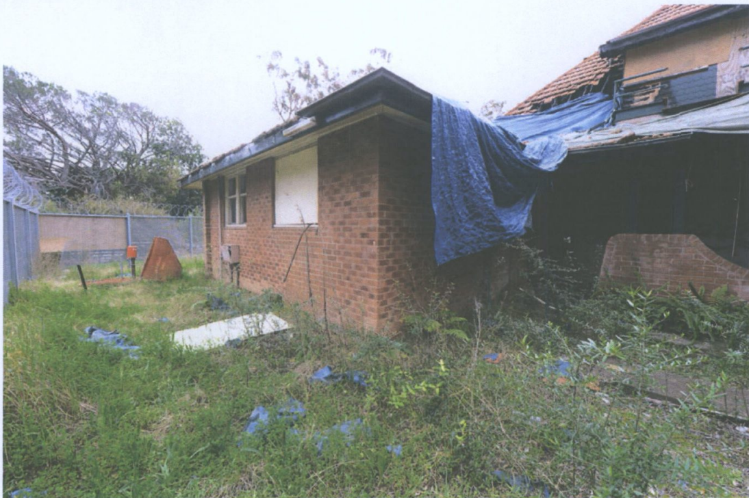
Figure 33 The rear of the former garage building with fire damage in the background. This building has been reworked and was an addition. There is considerable scope to redevelop this part of the site including replacing the current wing to allow discrete new development on the site. Such a wing could accommodate additional rooms and garaging. Removing part of the far embankment could also be considered without compromising the heritage values of the place. Paul Davies 2014.
