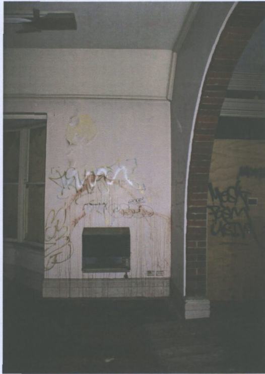
Figure 21 The main entrance (Hall 1) and reception room facing north, note loss of render to archway. Paul Davies 2014.
