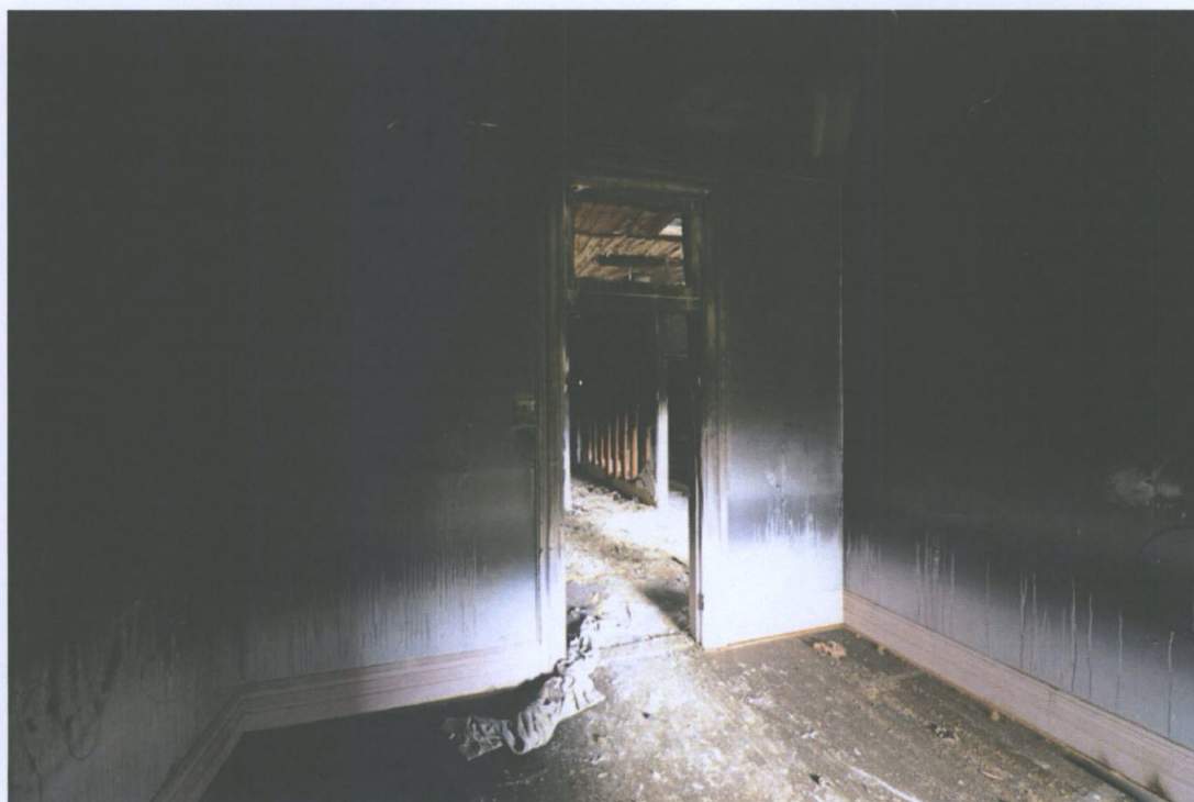
Figure 30 Room xxx showing impact of smoke and heat damage. It is likely that the wall finish to the right and ceiling will be fire damaged behind the plaster linings and will require replacement. Paul Davies 2014.
