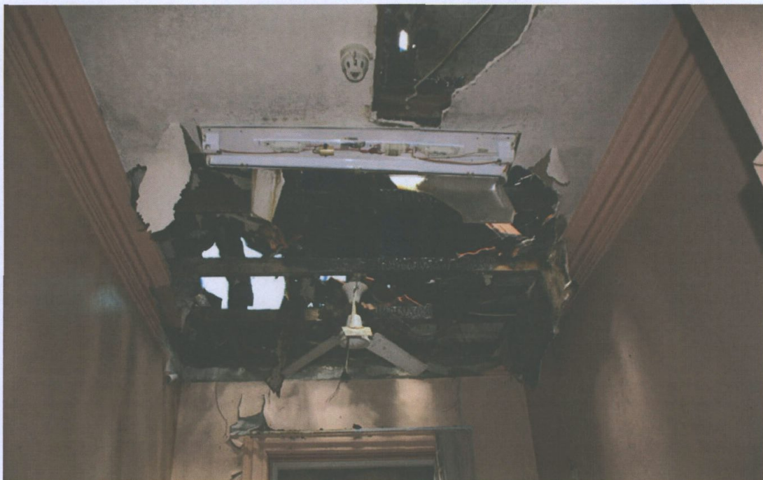
Figure 16 Damage to the ceiling of Room 6 from the fire revealing the pressed metal ceiling above the lowered plaster ceiling. Paul Davies 2014.
